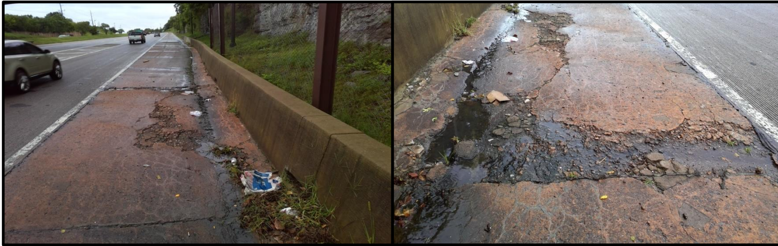
Possible faulting and subgrade issues
