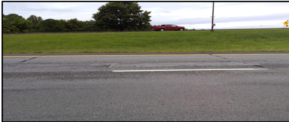
Asphalt overlay on concrete deteriorating
